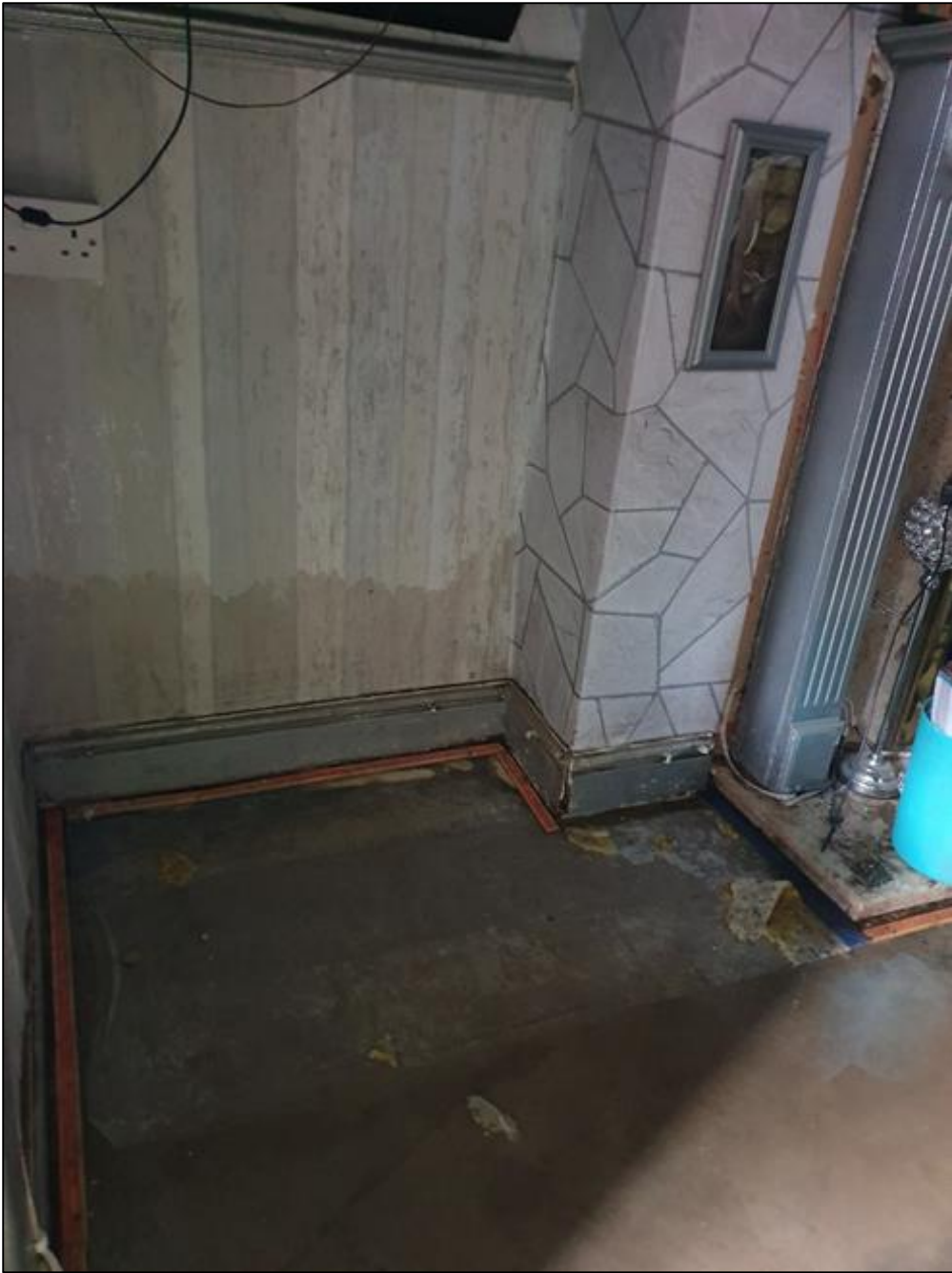
Photograph 3 Flood damaged living room of property in Meadow Street. Damaged carpets have been removed and the water mark left by the flood waters can clearly be seen. (February 2020).
